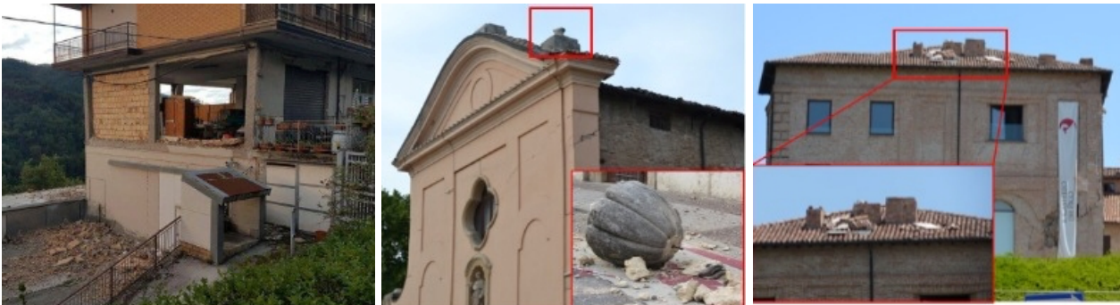
Figure 1. Post-earthquake damage to NSCs in reinforced concrete and masonry buildings.
